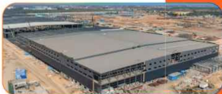
Home to India's First Lithium-ion Battery Manufacturing Giga Factory, Sanand
